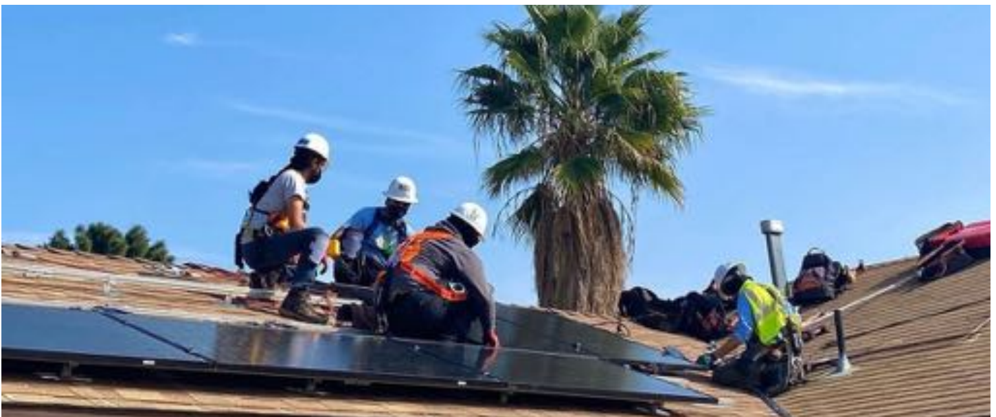
GRID Alternatives Solar Installation on a resident's home in Pacoima on March 2022 . Source: GRID Alternatives GLA
