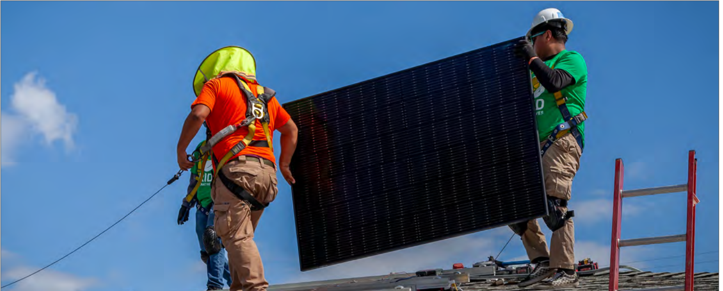
GRID Alternatives staff and high school students install rooftop solar panels in the project area. Photo credit: GRID Alternatives
