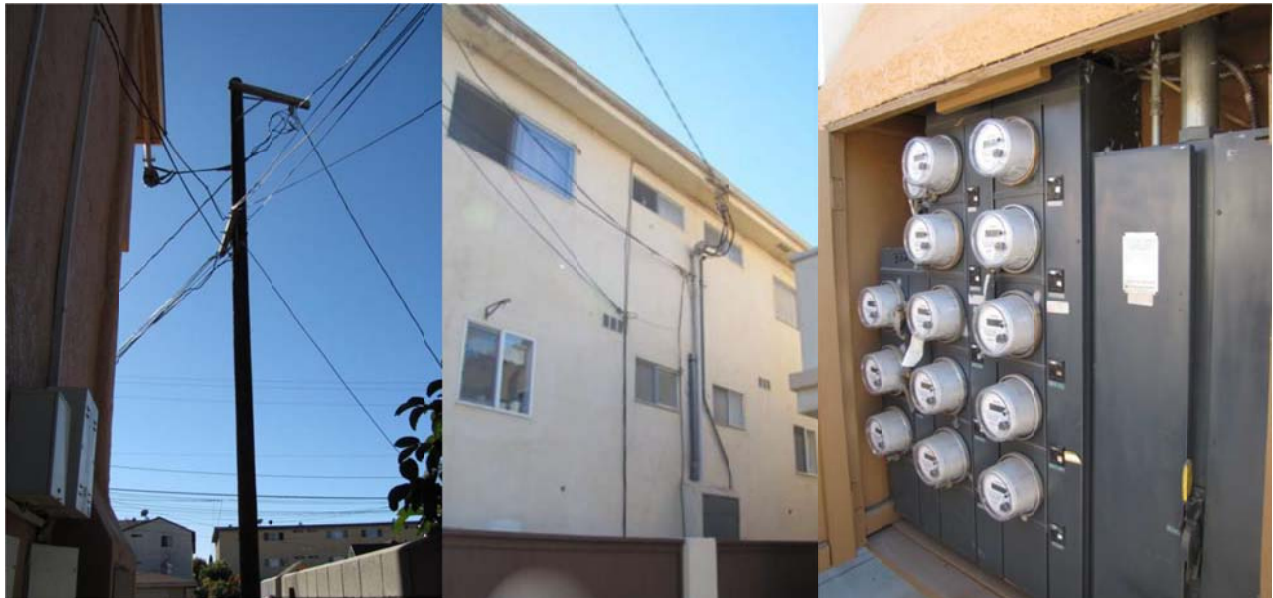
Figure 4.2: Photos of Overhead Service Drops and Meters at MUDs
