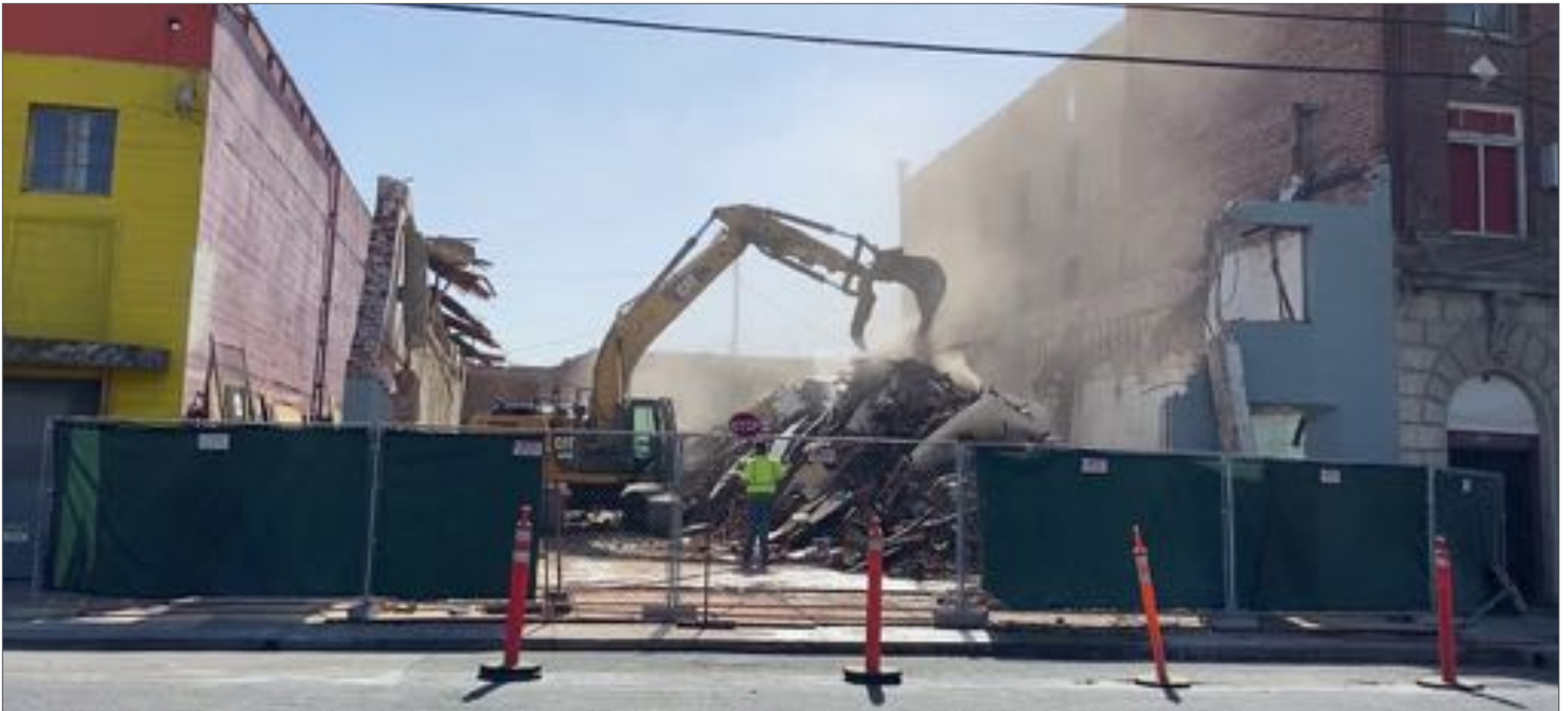
Demolition of Razil Social Cub, a culturally significant building in Stockton’s historic Little Manila district, after financing could not be secured for structural repairs. Photo credit: Little Manila Rising
