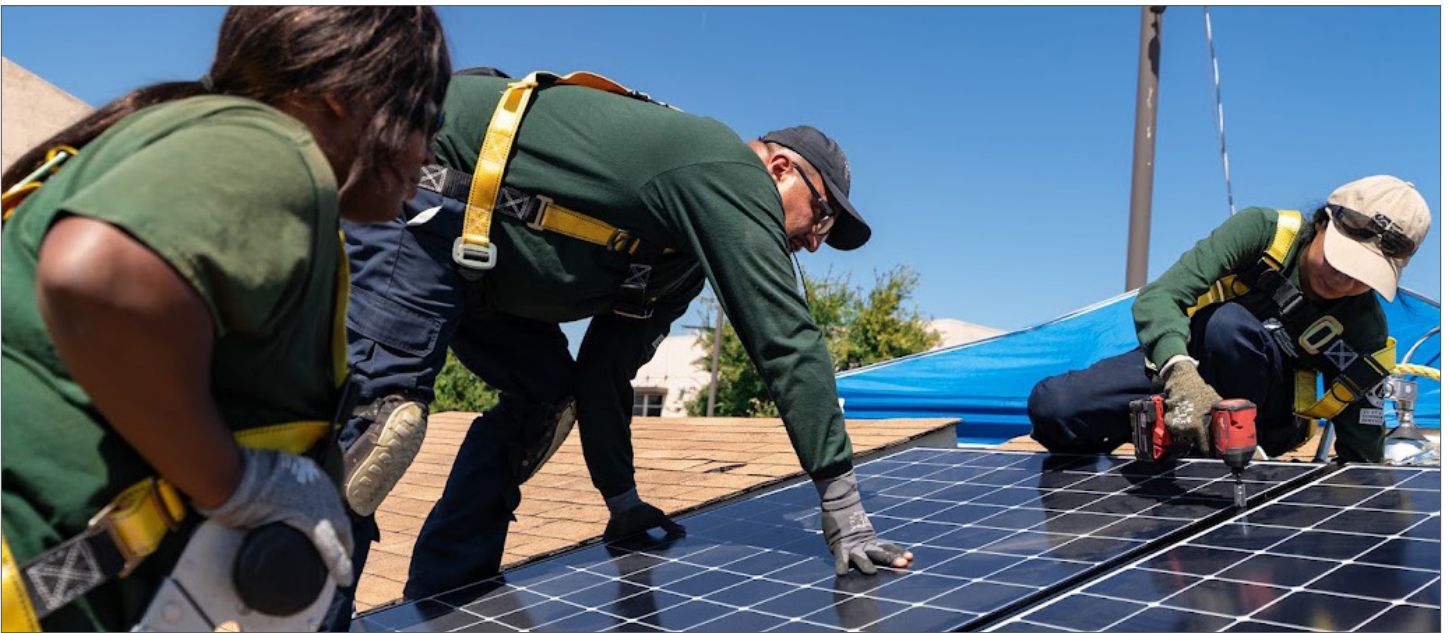
Workers from Fresno EOC install new solar panels on a residence. Photo credit: Transform Fresno
