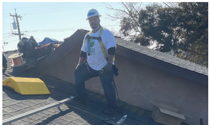
Matthew De La Rosa working at installation project job sites in Fresno. Photo credit: GRID Alternatives
