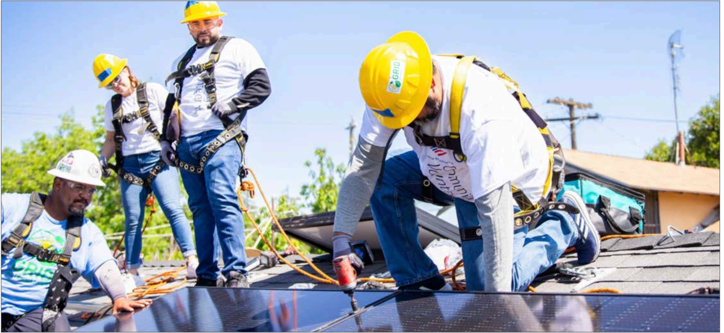
GRID Alternatives' volunteers installing rooftop solar panels on a residence. Photo credit: GRID Alternatives
