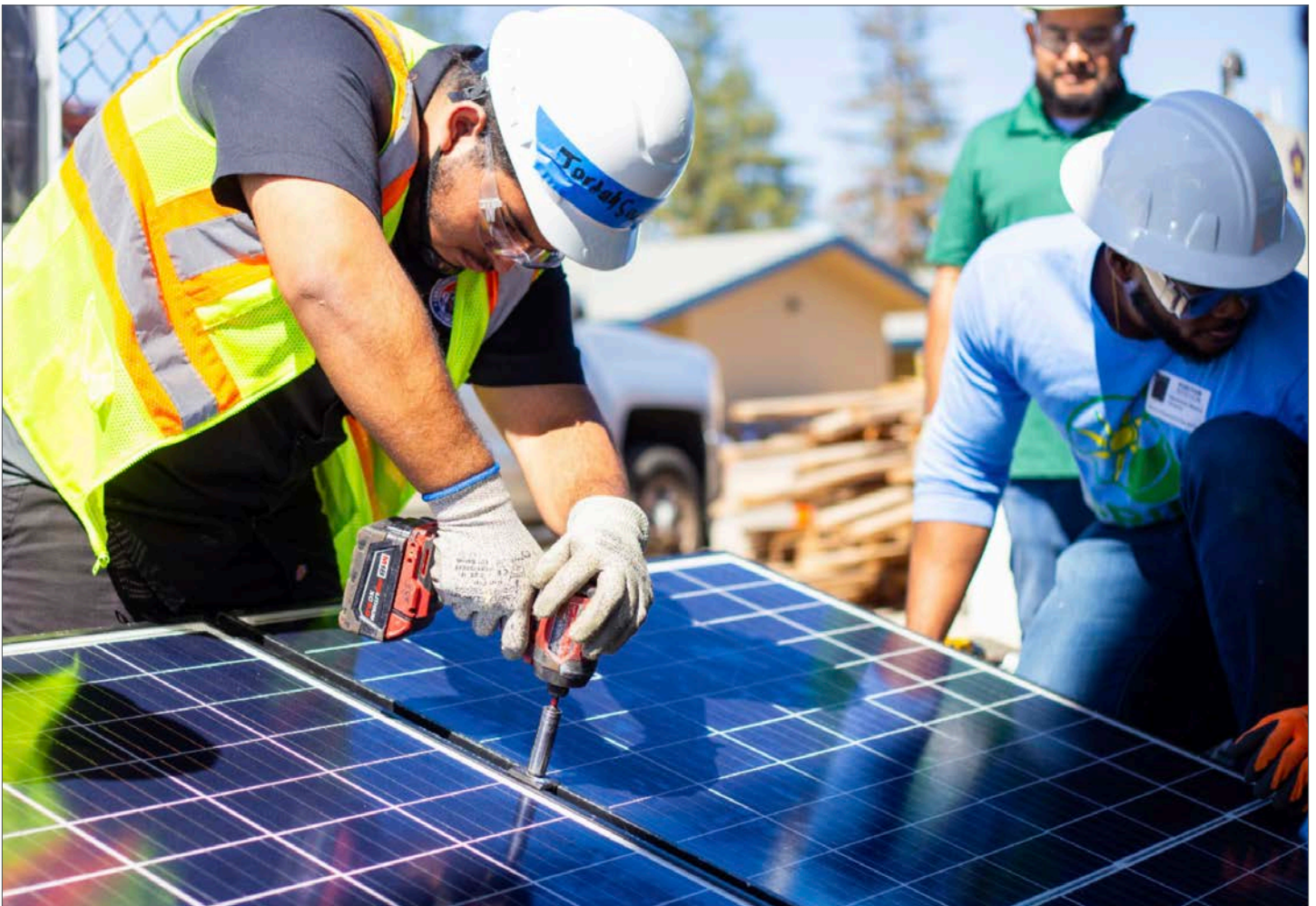
GRID Alternatives' volunteers install solar panels as part of their job and skill building training. Photo credit: GRID Alternatives
