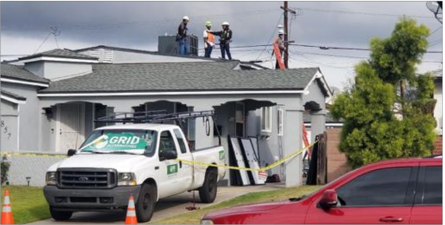
GRID Alternatives LA installing solar panels on a Watts home September 2021. Photo credit: GRID Alternatives Greater Los Angeles
