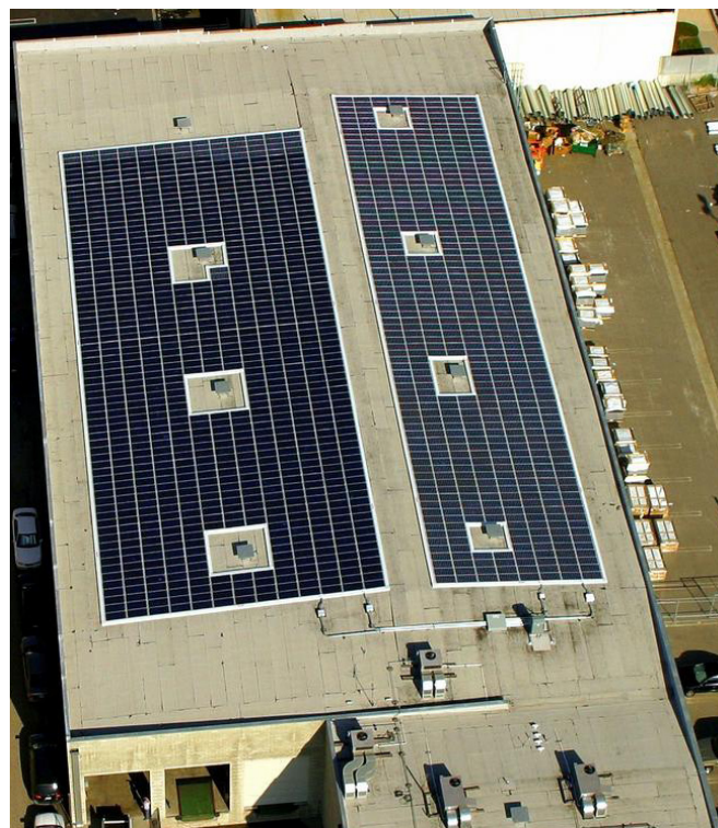
A 106 kilo-watt rooftop solar system. Under current market conditions, this system costs over $600,000.
