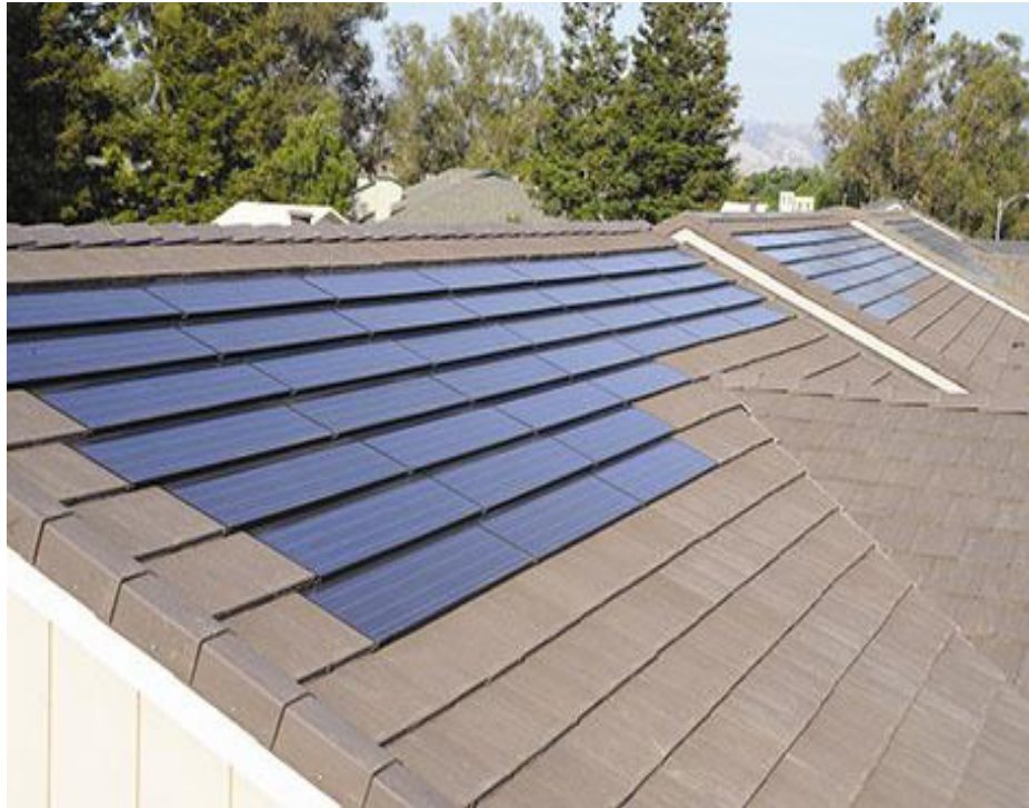
A specific application of solar technology
