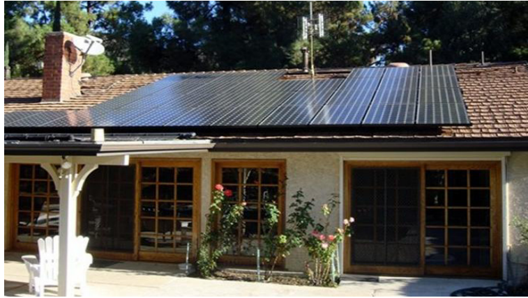
A 7 kilo-watt residential solar system
