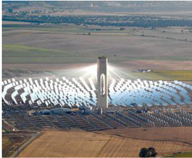
A large solar thermal power plant in Spain.
