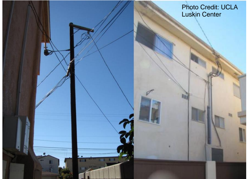
Two examples of overhead service drops providing electricity to the MUD's electric box
