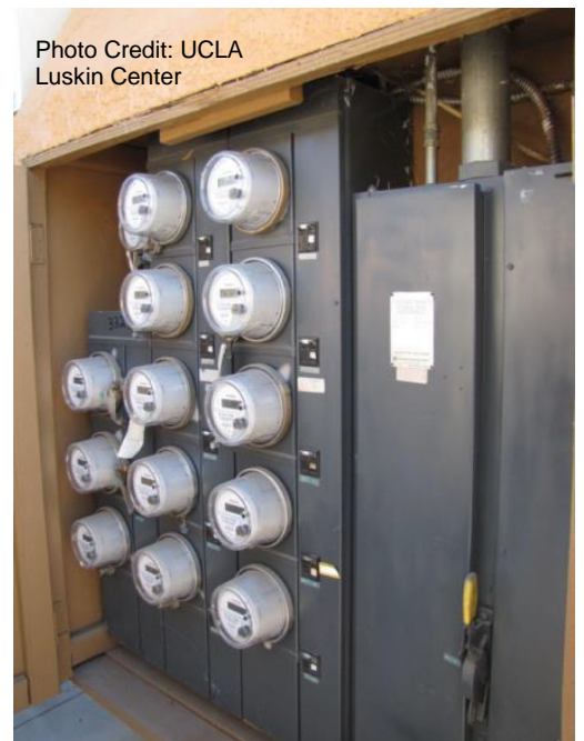
A grouping of house and unit meters (i.e. the meter section) and their main breakers inside an electric box.
