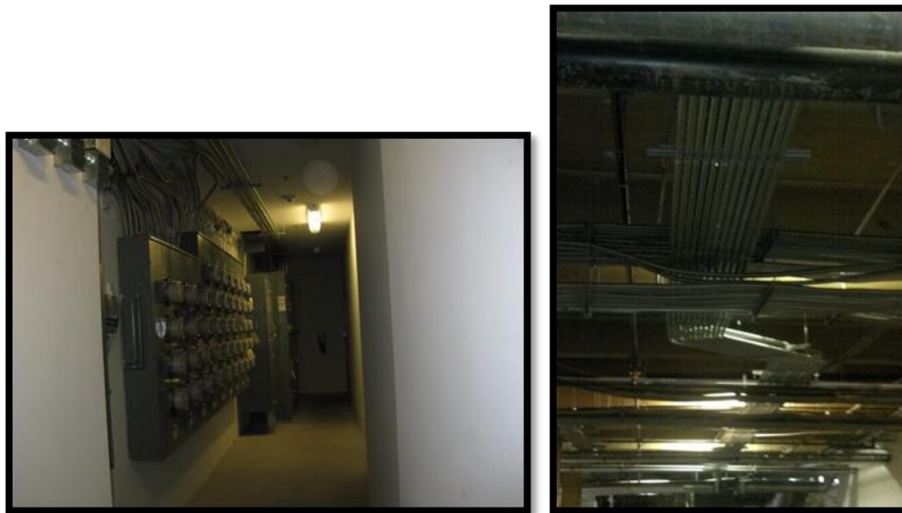
Figure 14. Electrical Room and Conduit for Case Study 2
