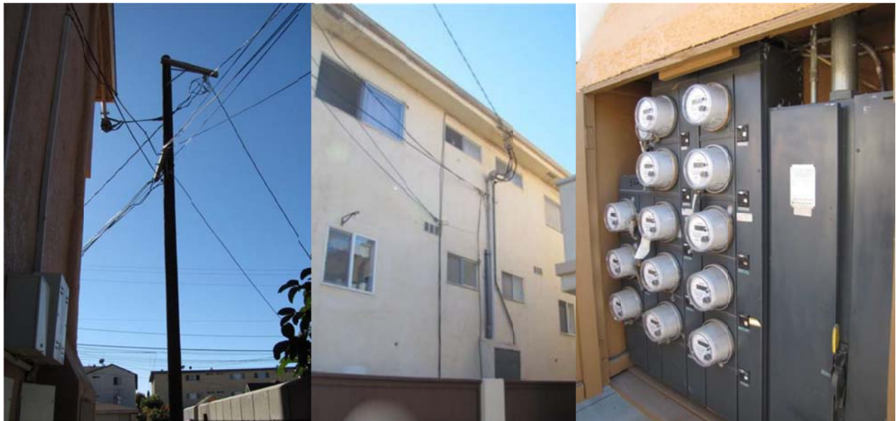
Figure 20. Photos of Overhead Service Drops and Meters at MUDs
