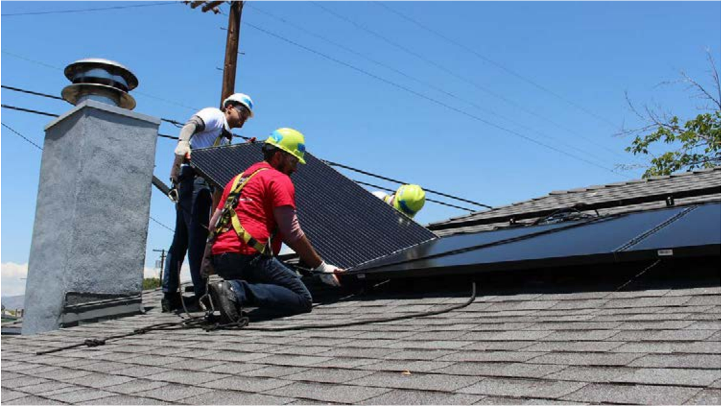
Rooftop solar PV panels installed by GRID Alternatives staff and trainees in Los Angeles. Photo credit: GRID Alternatives
