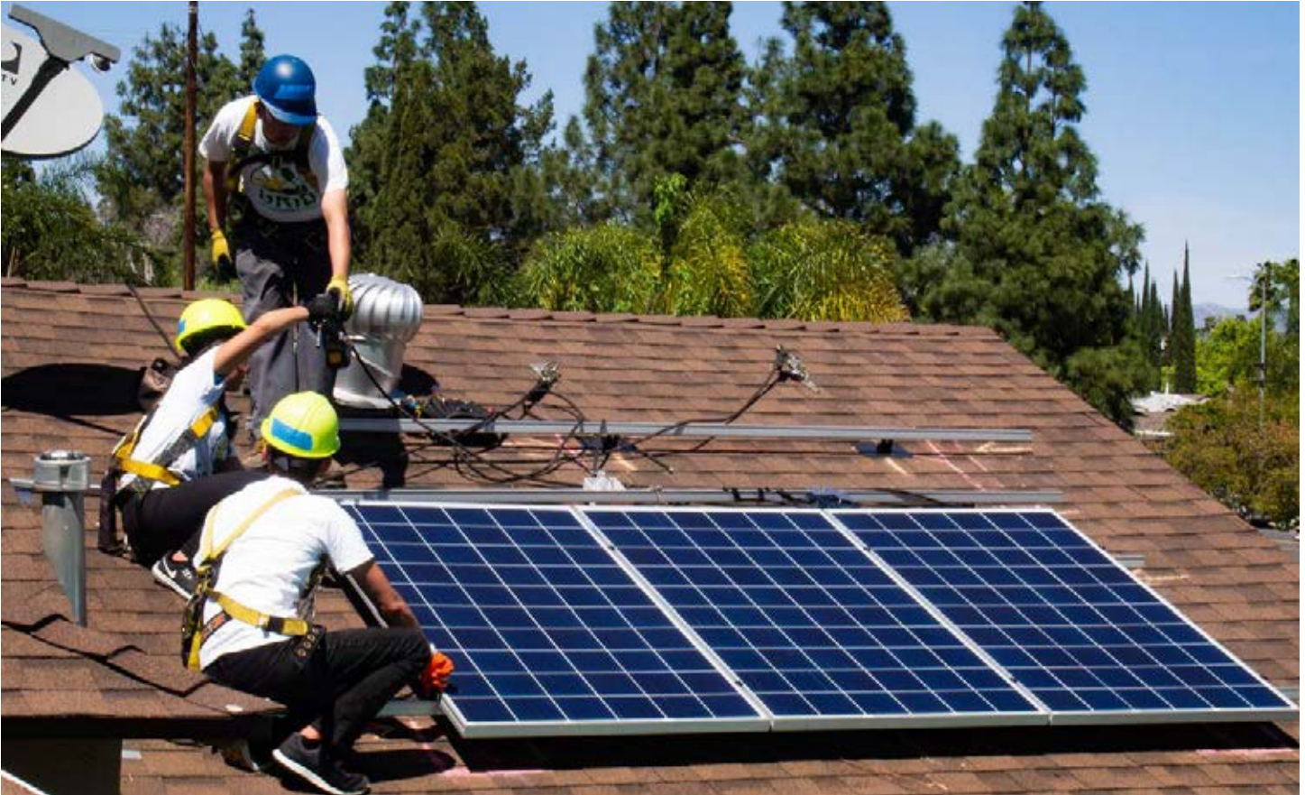
GRID Alternatives solar installation trainees in Los Angeles. Photo credit: GRID Los Angeles
