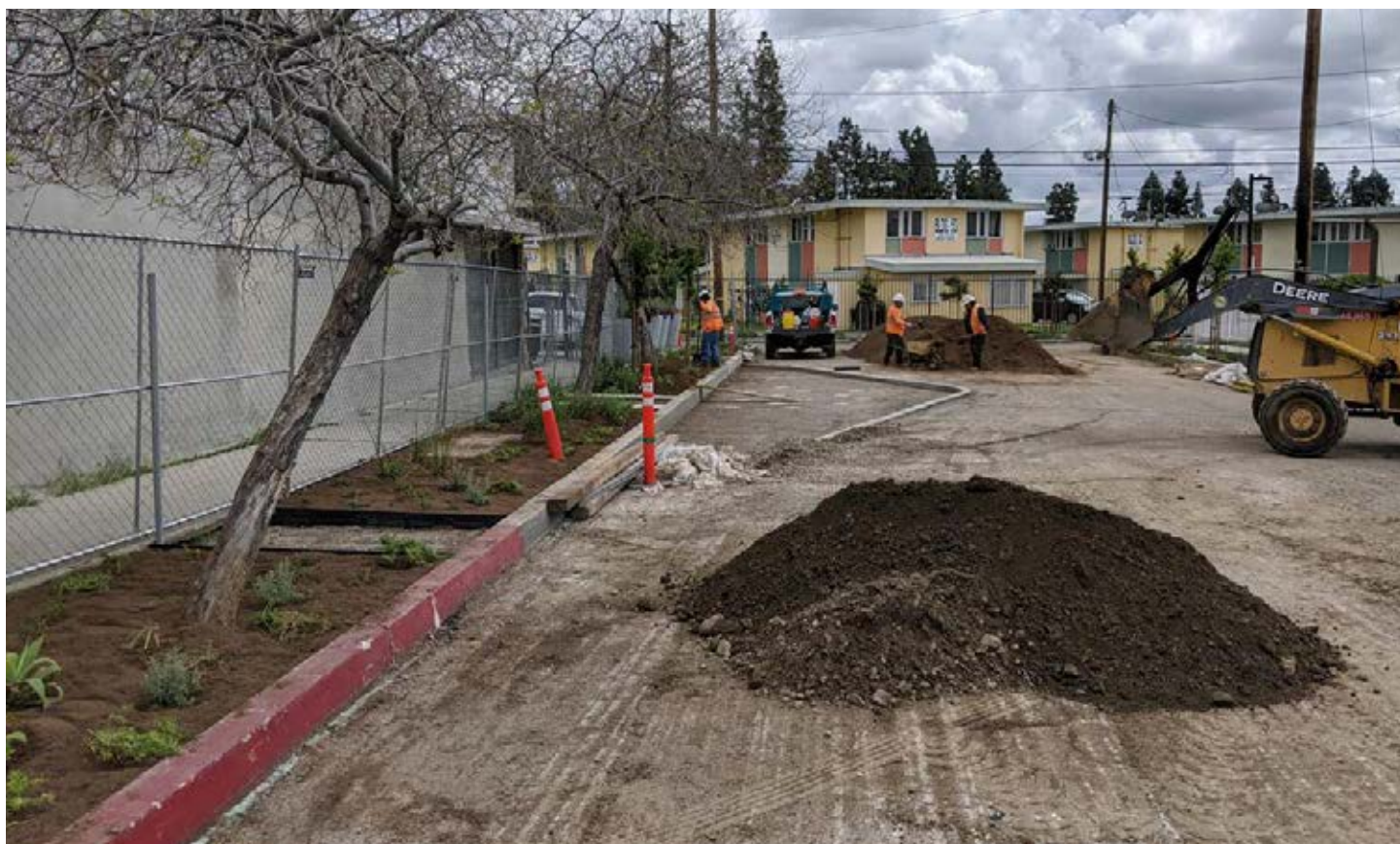
Construction at Bradley Green Alley and Plaza, which will receive a number of improvements as a result of a leveraged project. Photo credit: The Trust for Public Land, April 2020.
