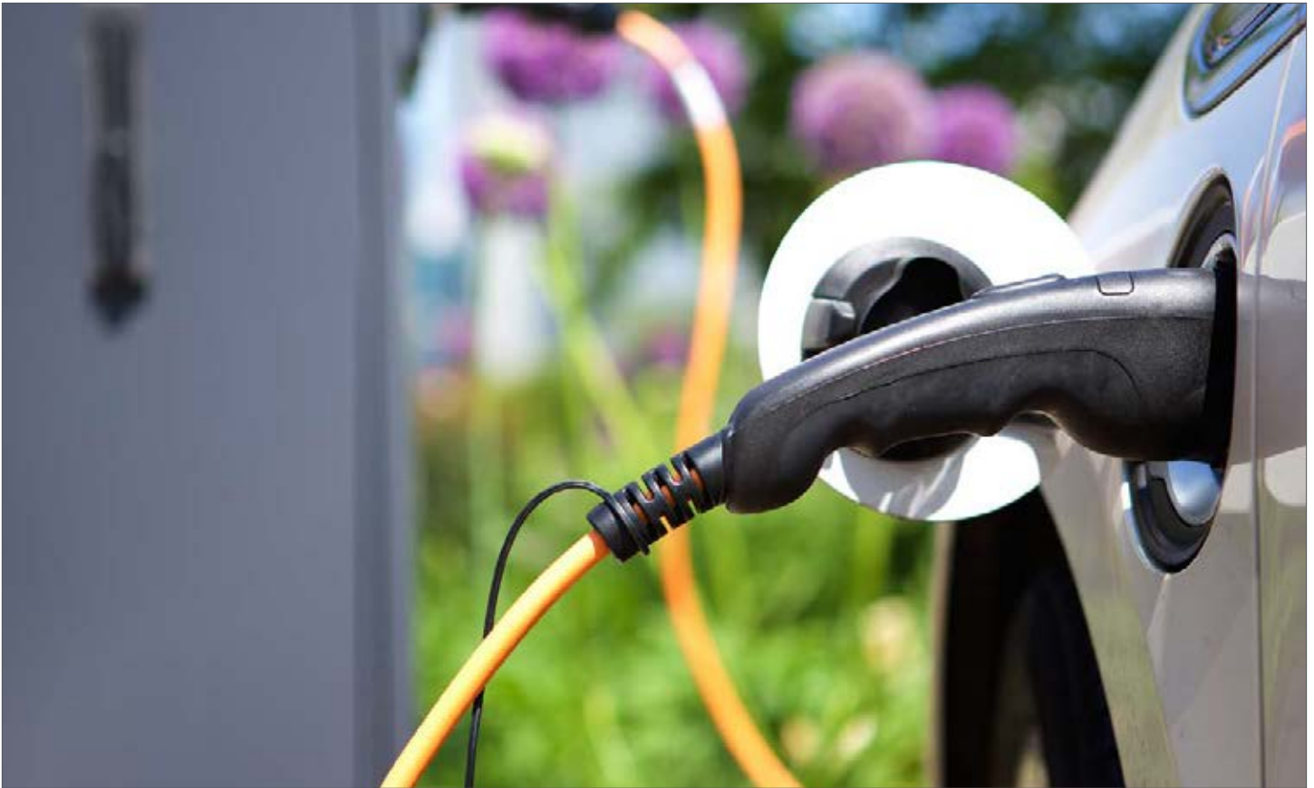
The Electric Vehicle Charging Station project will install critical infrastructure at four mobility hubs.
