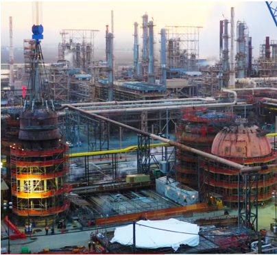
FCCU at Chevron Richmond Refinery
