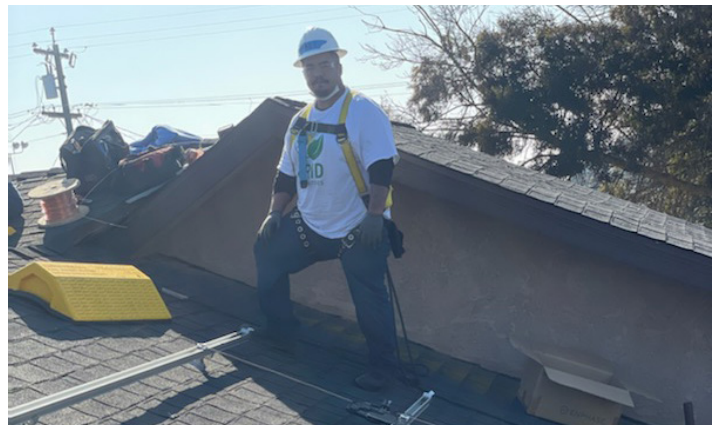
Matthew De La Rosa working at installation project job sites in Fresno. Photo credit: GRID Alternatives
